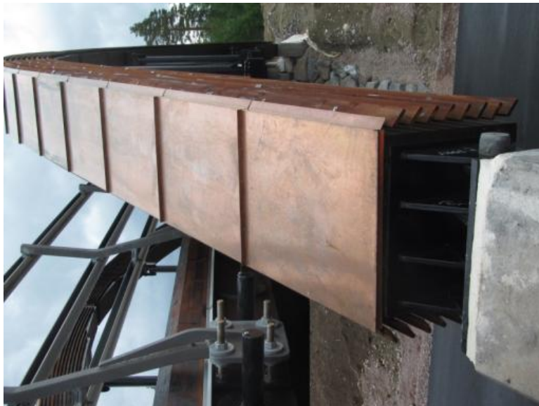
Figure 5. Copper flashing, louvres and drainage promoting connection on Åset Bridge in Norway, built in 2014.
