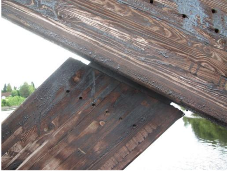
Figure 6. Wood components spaced apart by metal connectors on the Flisa bridge in Norway.
