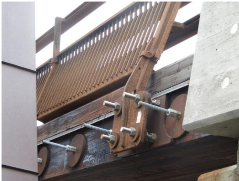
Figure 7. Metal plate connectors not too large to prevent drying on Sletta Bridge in Norway.
